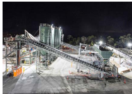
Boral's mobile concrete batch plant at Mount Kuring-gai, NSW, for the NorthConnex motorway in Sydney (estimated completion 2019)
