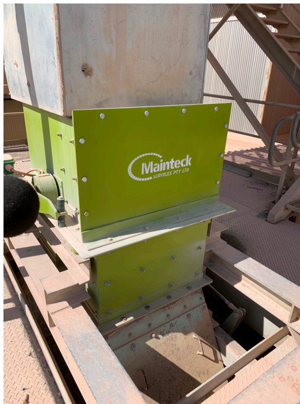
Photograph 3.2: Magnet impact plate on RM7 roof platform
